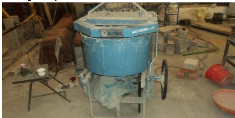
Fig V: Concrete Mixing Machine
