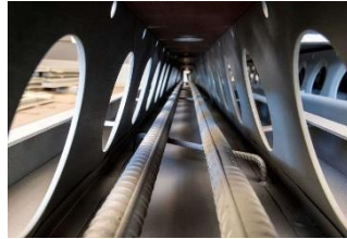
Figure 9: Fire Rebars Inside Deltabeam
