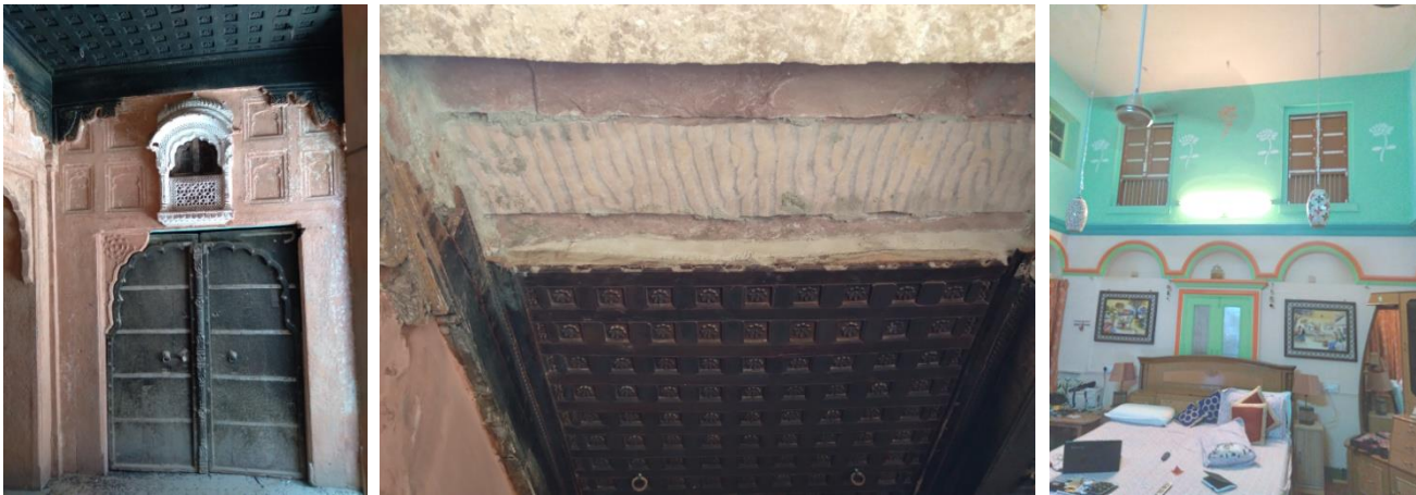
Fig 10a,b & c Ceiling is made out of slabs as shown and covered with wooden false ceiling for better insulation. In 10c double height room can be seen with windows for proper ventilation (Source: Author)
