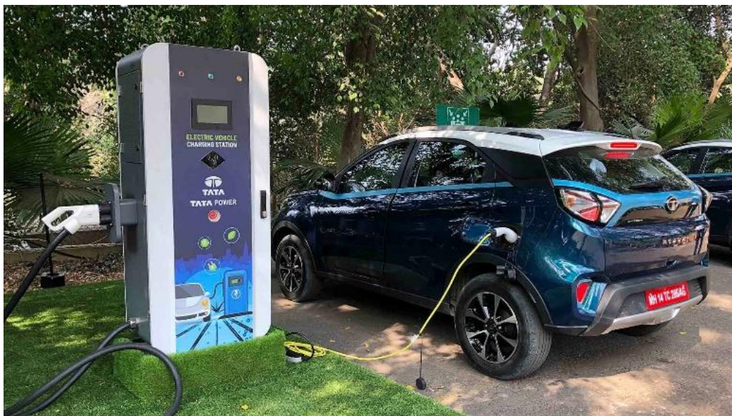
Fig no 05 Tata charging device
