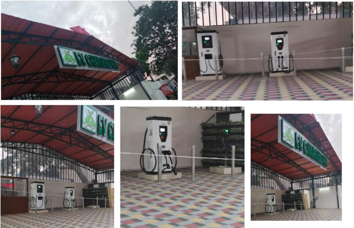
Fig no07Yeshwanthpur Charging Station
