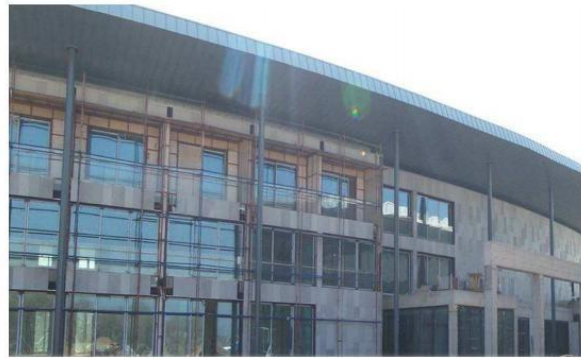
GFRC Panels used for heat insulation
