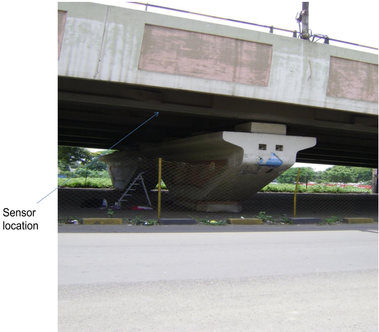
Figure 2: Sensor location on Seven Hill bridge
