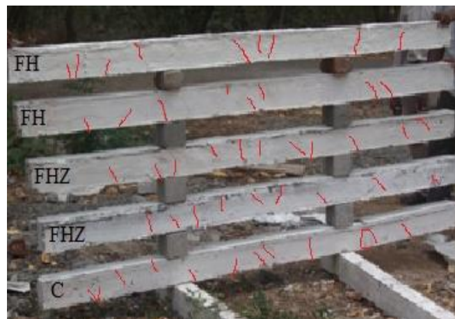
Fig.4.12 Failure pattern for all the beams.
