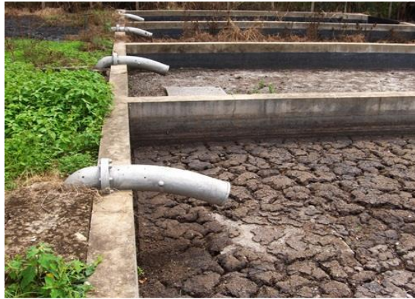
Fig.7 Sludge Thickening Unit
