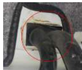
Fig. 5- Hose fouling with sharp edge
