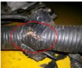
Fig. 4 - Damage due to sharp edges
