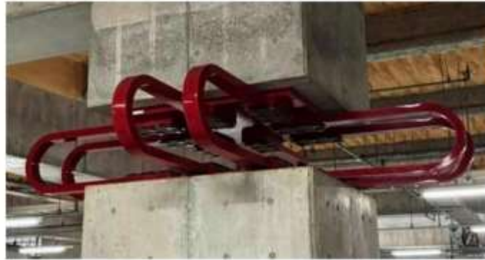
Fig. No. 3.3 Metallic Seismic Dampers in RC Columns
