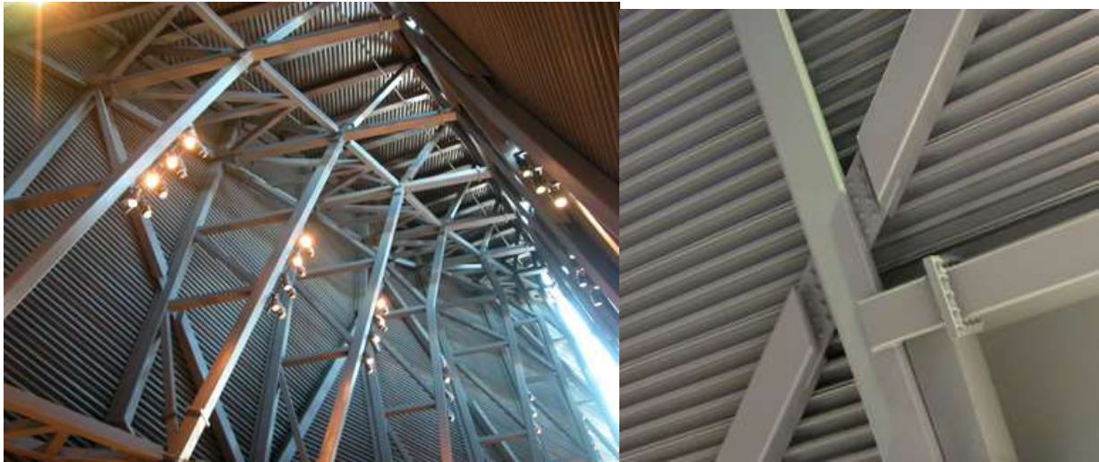
Fig.5 ‘The Canadian War Museum in Ottawa uses AESS. Due to the irregularity of the structure, tight tolerances are required. The profiled decking is also left exposed to view’ (Boake, B.E.S., B.Arch., M.Arch., & AP, 2012).
