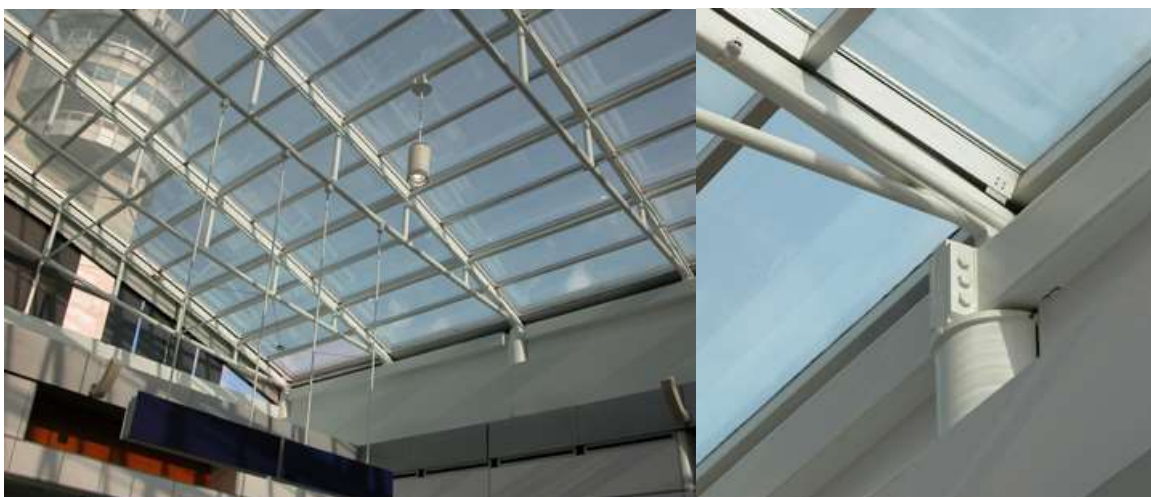
Fig.3 ‘Pierre Elliott Trudeau Airport, Montreal: The trusses supporting this skylight are quite characteristic of AESS 2 type steel. The viewing distance is over 6 meters but the design needs something more than a standard joist or truss. The detailing is simple, and the viewer is not close enough to see the texture of the connection, only the form of the truss’ (Boake, B.E.S., B.Arch., M.Arch., & AP, 2012).
