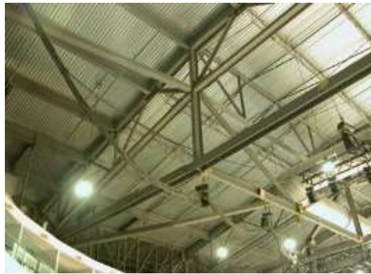
Fig.2 ‘Ricoh Centre, Toronto, ON: The trusses that span the arena proper in the Ricoh Centre, given their roughly detailed design style as well as the less refined nature of the space’ (Boake, B.E.S., B.Arch., M.Arch., & AP, 2012).
