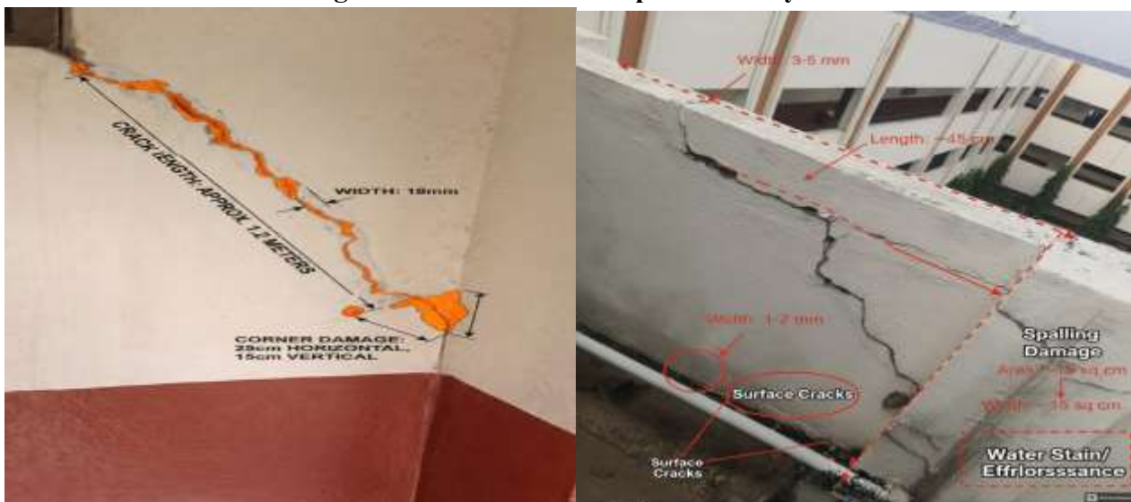
Figure 2: Visual Crack Inspection analysis
