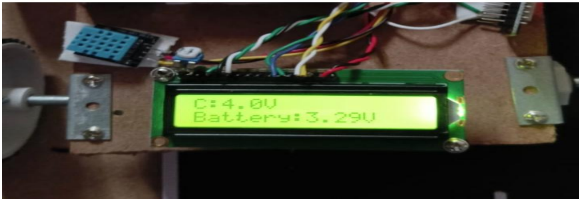
Fig 8.3: Battery voltage has increased to 3.29V, confirming that wireless charging successfully transferred power.
